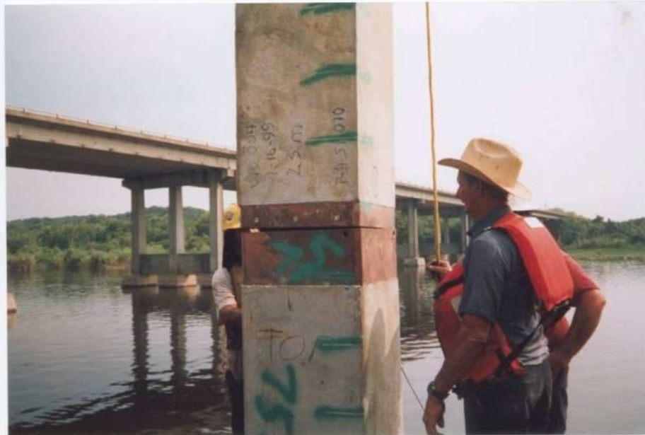
24" sq. Sure-Lock Pile Splice – FDOT St. John's River Bridge. Top pile segment lowered so splice plates fit together.
