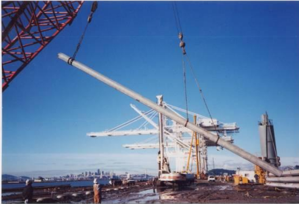
24" oct. Sure-Lock Pile Splice – Port of Oakland, Berth 57, 2001 Bottom pile segment of 80 ft. with Female splice half lofted.
