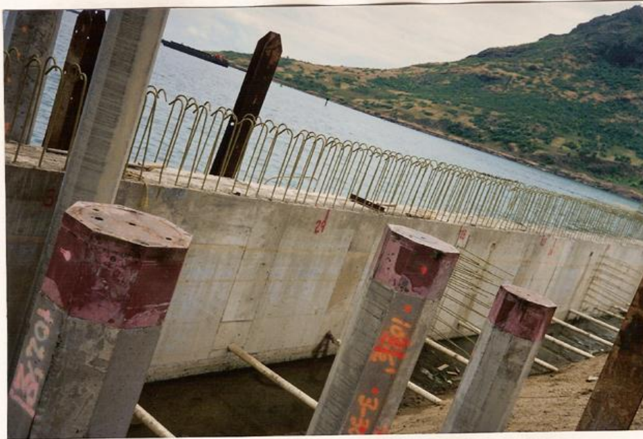
650 – 20" octagonal piles for Kauai Pier 3. Splices connected 2 – 100 ft. segments for 200 ft. piles. Bottom segments shown with driving plates. Second segments then spliced and driven with a production rate of 10 piles per day.
