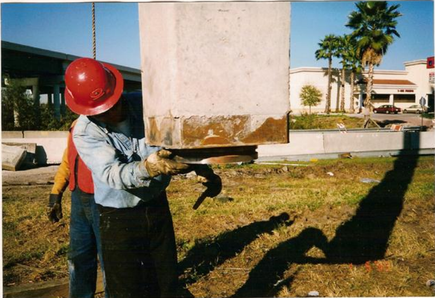
Top pile segment with circular Male plate, lofted, cleaned off, and ready for splicing.
