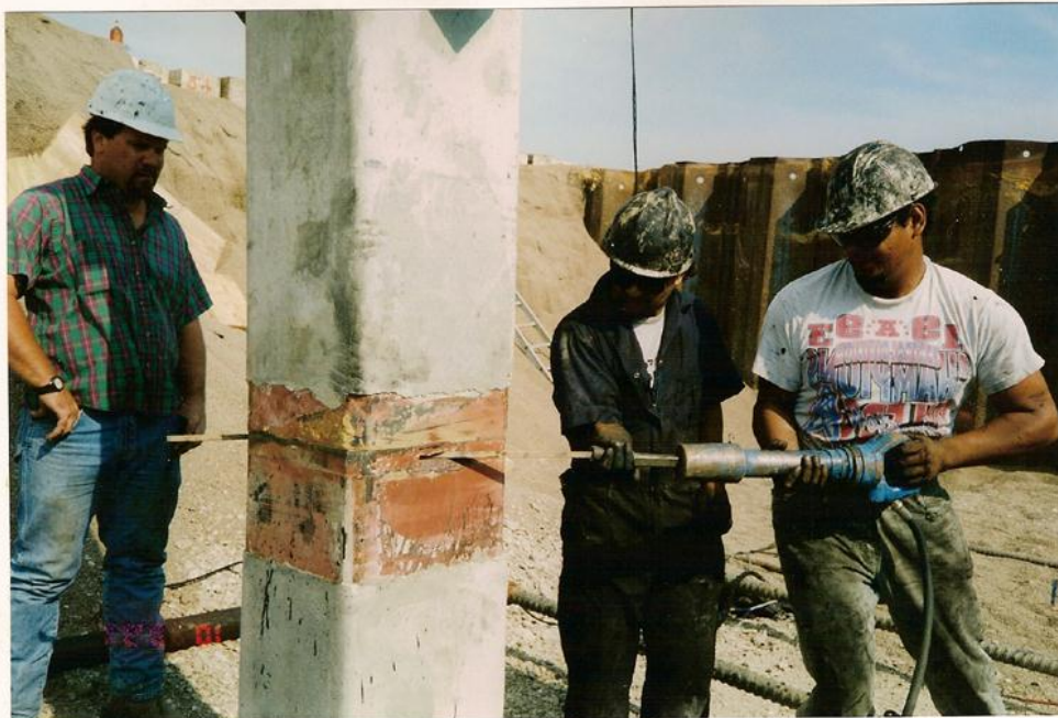
16" sq. Texas DOT wharf – 2 locking bars driven into the splice grooves to form a circular shear key – in less than two minutes.
