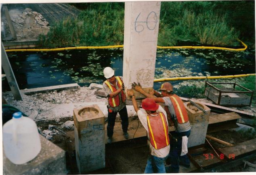
18" sq. Splice for FDOT bridge widening project near Orlando. Bottom segments with Female splice half driven first.
